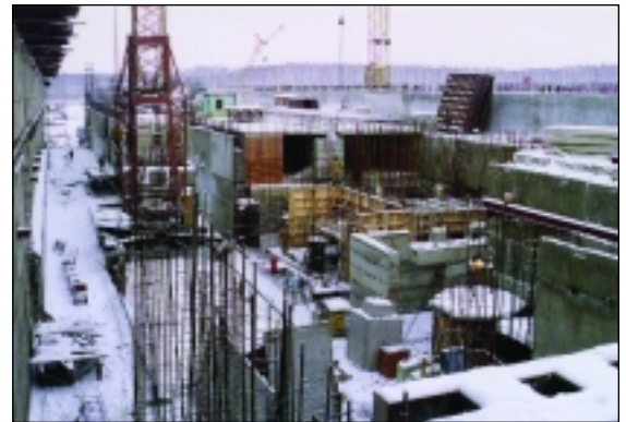
Mayak Fissile Material Storage Facility under construction at Ozersk, Russia. (photo courtesy of DTRA).
